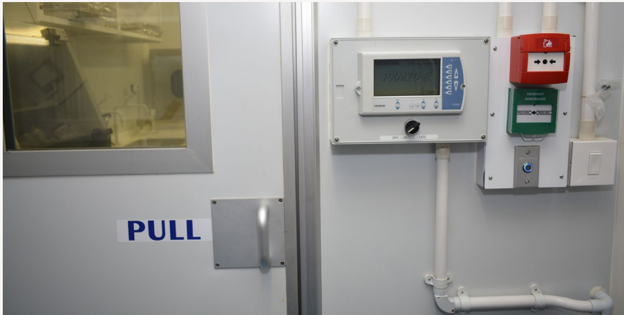
Control Panel of the BSL-3 lab (Photo credit: Samuel Murmu, CTB)
