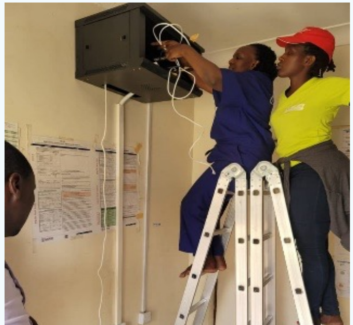
District representatives installing and configuring network routing and switching equipment at Namuyanja HC IV in Isingiro district.
