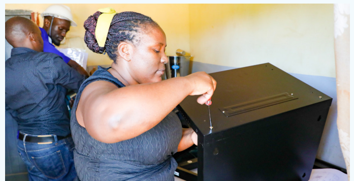
SSCS and Mpigi District government staff preparing to install a wall-mounted network rack at Kituntu HC III in Mpigi District.
